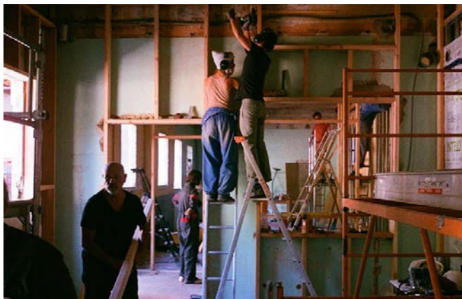
Fig 2. La Place des Possibles, Saint-Laurent-en-Royans, France. A moment of the participatory construction workshop organized for the redefinition of the spaces of the “Place des Possibles”. Photo: http://www.collectifetc.com/realisation/la-place-des-possibles/
