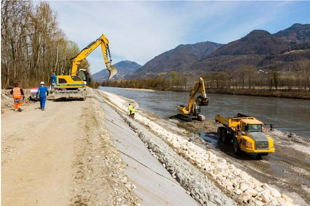
Figure 1. The project "Isère en amont" completing the bank protection in a sector of the project. Primarily driven by a quest for better flood management, the project struggles to truly integrate the river as a major component in territorial development. Source : Symbhi/SO Dupontrenoux (2018)
