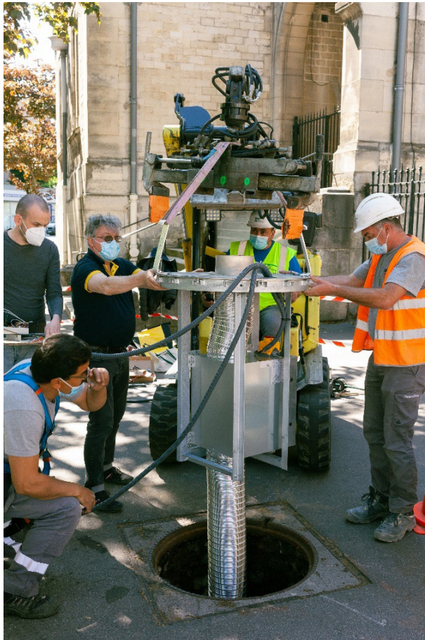
Figure 1/Figura 1. Installing and programming of the engine. Source: Alt 2021
